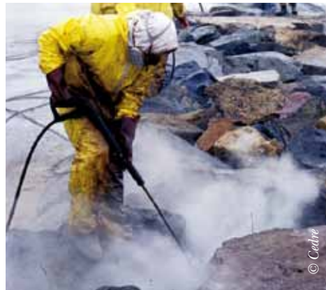
Risks of pollutant splashing
