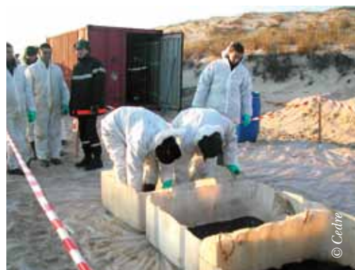
Successive tanks for rough and intermediate cleaning
