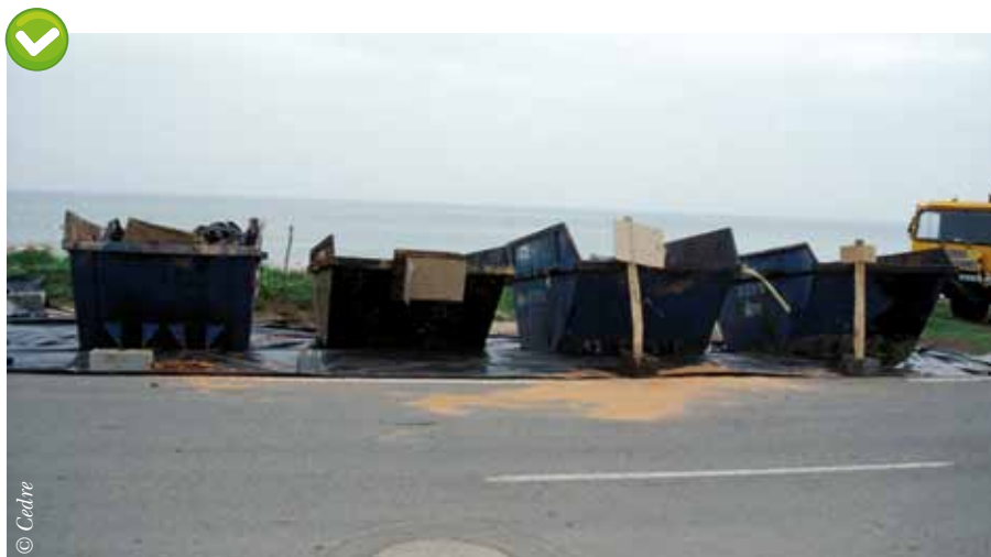
Skips for segregated waste storage
